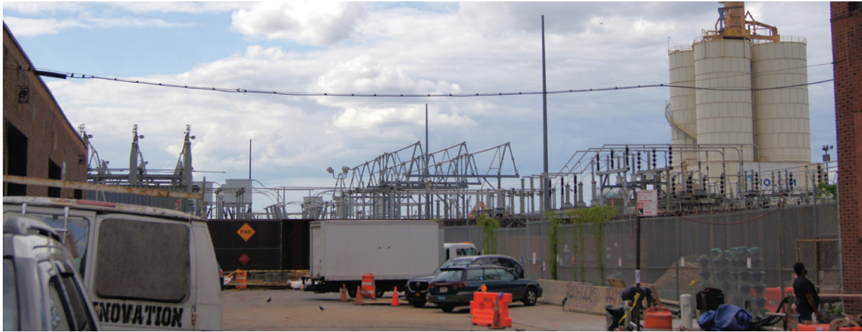
The Gowanus substation in Sunset Park is located next to the Gowanus generating station and the Joseph J. Seymour power plant in Brooklyn. PHOTO: SEBASTIAN BAEZ/UPROSE
