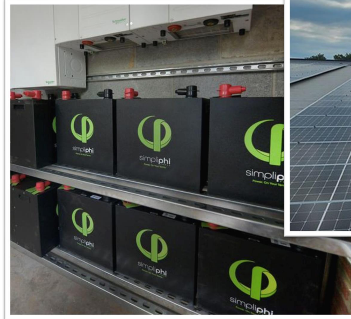
SimpliPhi batteries at Maycroft Apartments. Credit: SimpliPhi Power
