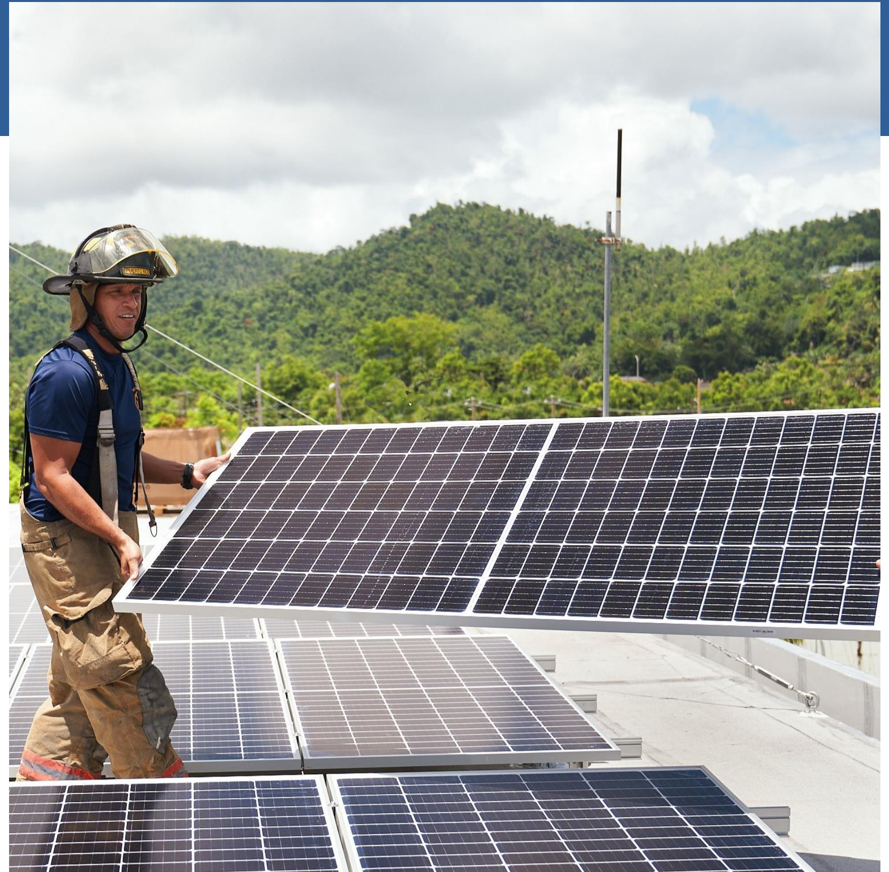
Solar installation in Puerto Rico. Credit: Solar Responders
