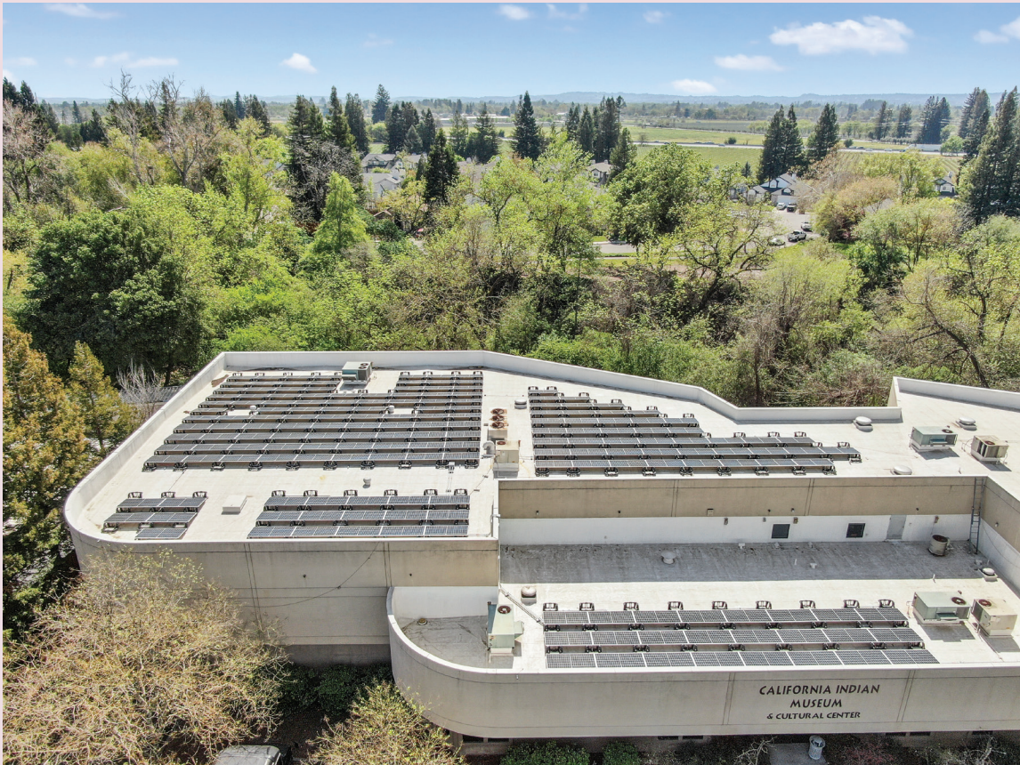
California Indian Museum and Cultural Center, Solar Array.
