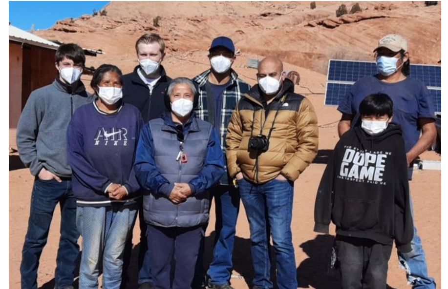
Navajo Nation residents install solar+storage for their off-grid home after receiving a TAF in 2021. Credit: JPHB, TAF engineering partner
